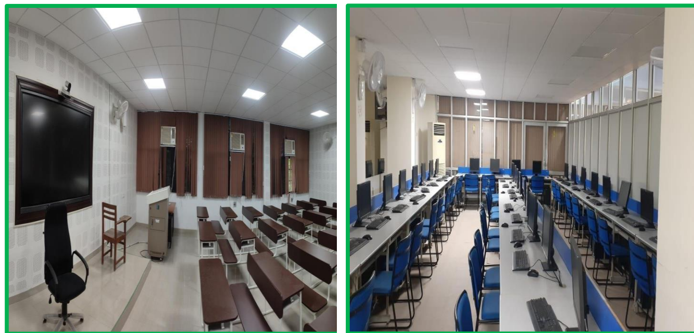
FIG 34 LED FIXTURES IN SMART CLASSROOMS (SCIENCE HALL 4, TF)
