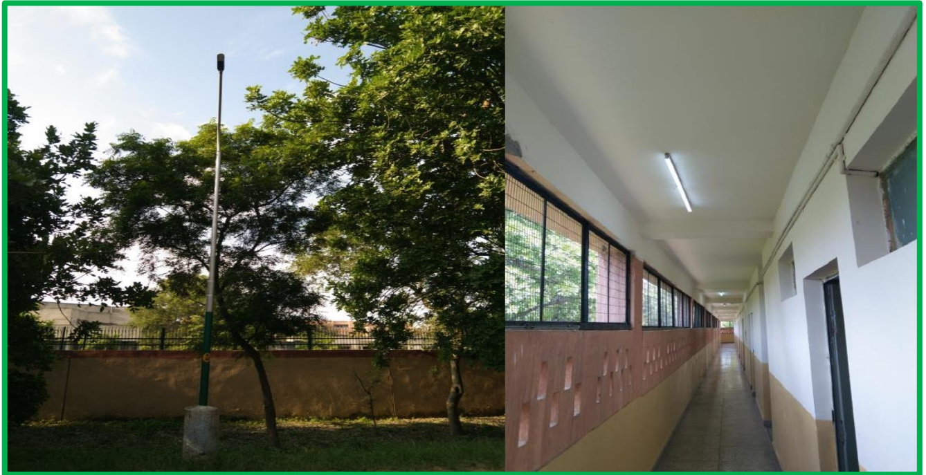
FIG 31 LED FIXTURE (STREET LIGHT, ROAD-A NEAR H POLE)/ LED FIXTURE IN GIRLS HOSTELNO.1, FF (CORRIDOR) NEAR ROOM NO. 231
