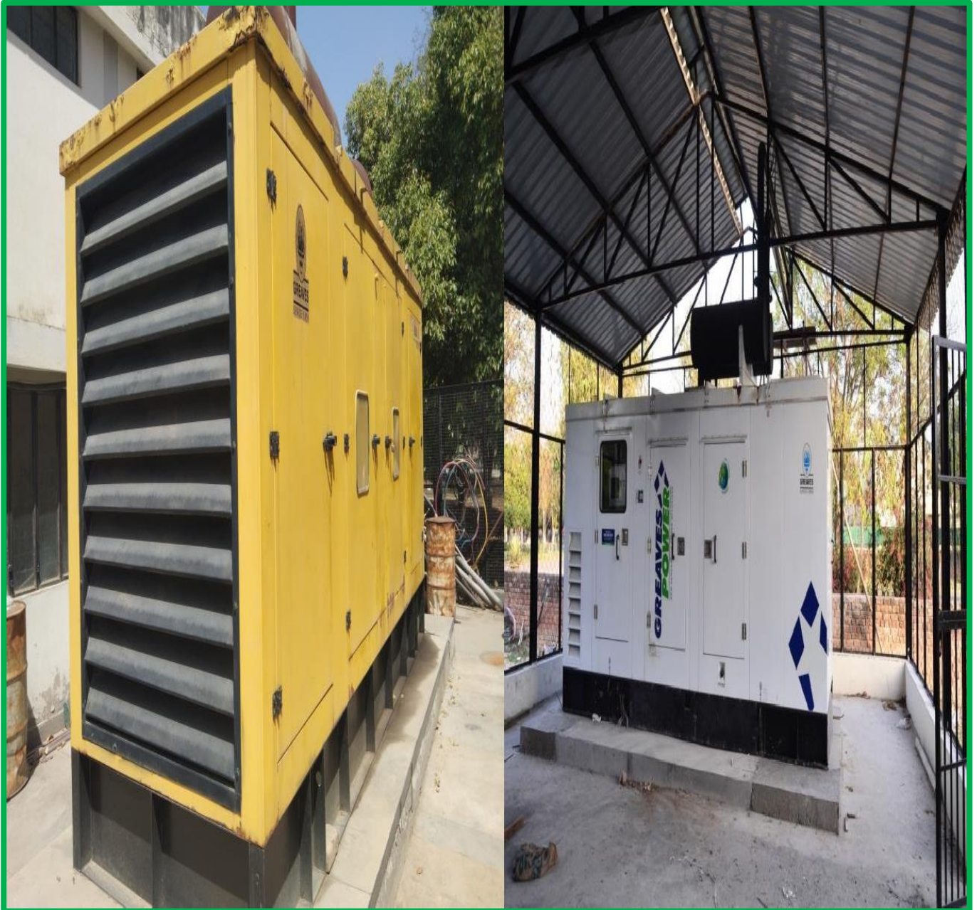
FIG. 40 DG SET INSTALLED IN ELECTRICAL WING AND ESTATE OFFICE
