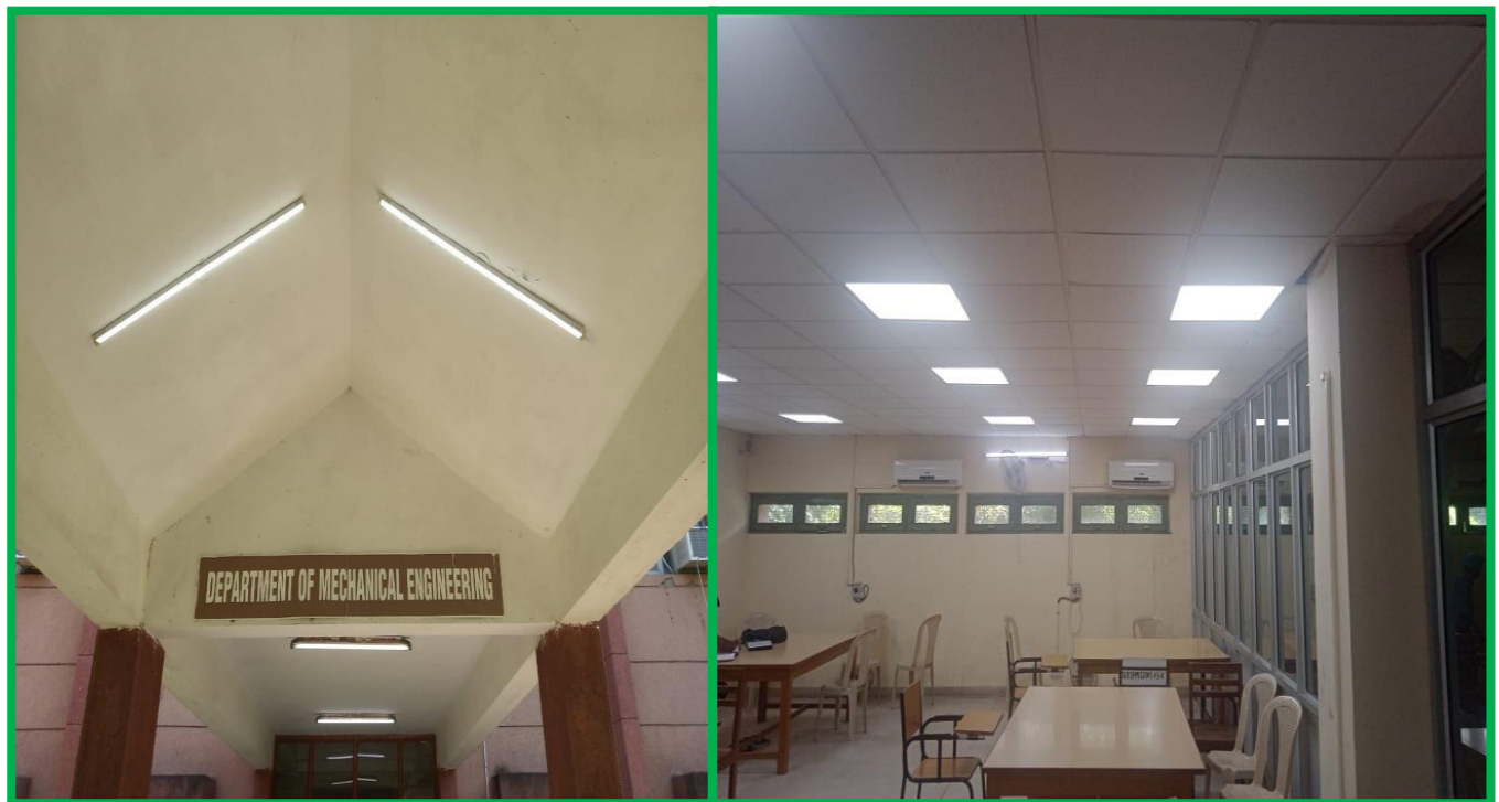
FIG- 32 LED FIXTURE IN ME ENTRANCE AND CENTRAL LIBRARY, FF (READING HALL)
