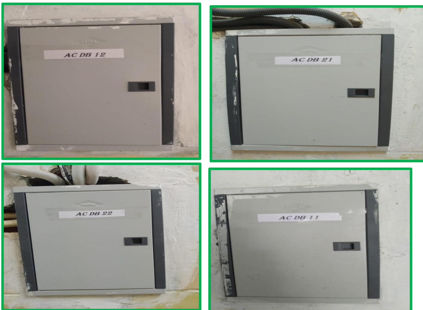
FIG 41 AC DB ATTACHED IN MECHANICAL BLOCK FOR ESSENTIAL AND NON-ESSENTIAL LOAD
