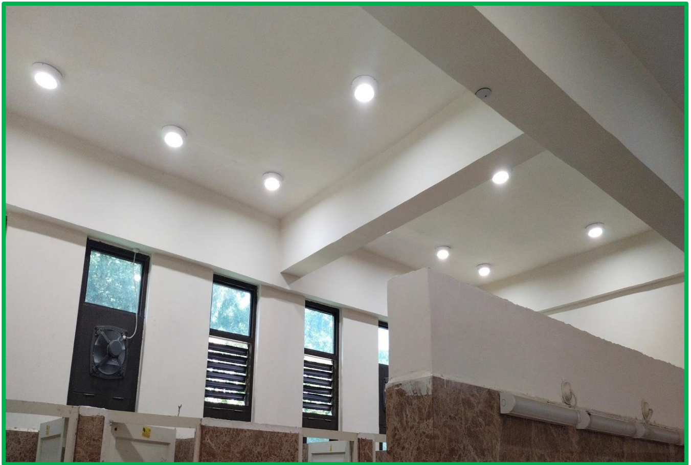
FIG 35 OCCUPANCY SENSOR INSTALLED IN THE WASHROOMS OF NEWLY CONSTRUCTED EDP BLOCK
