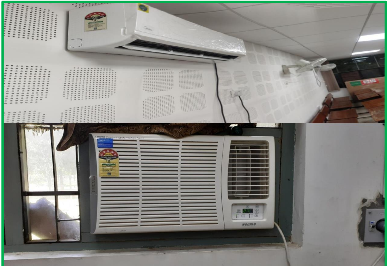
FIG .37 STAR RATED AIR CONDITIONING IN SMART CLASSROOMS (ME, M-117, GF)/ SMARTCLASSROOMS (HALL NO. 3, TF)
