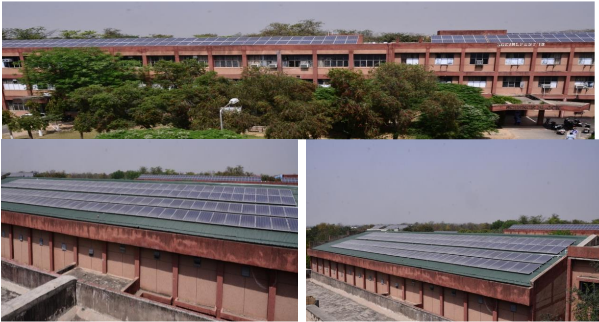
Fig. 3.11: Installed Solar Panel on the Roof Top of Buildings (Science and Mechanical Block)
