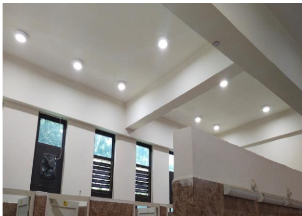
Fig. 3.7: Occupancy Sensor Installed in The Washrooms of Newly Constructed EDP Block
