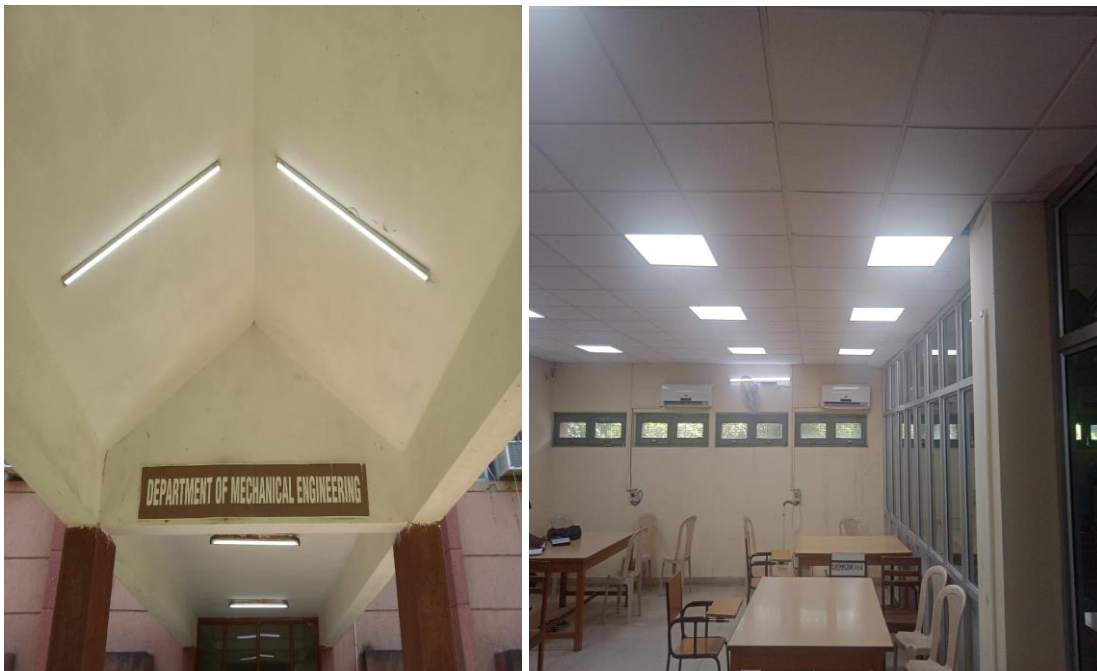
Fig. 3.4: LED Fixture in ME Entrance and Central Library, FF (Reading Hall)
