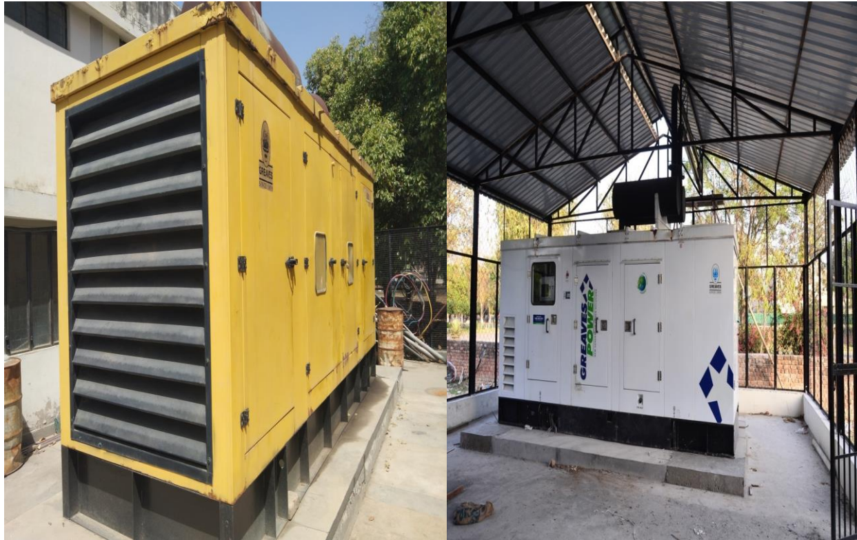
Fig. 3.12: DG Set Installed in Electrical Wing and Estate Office
