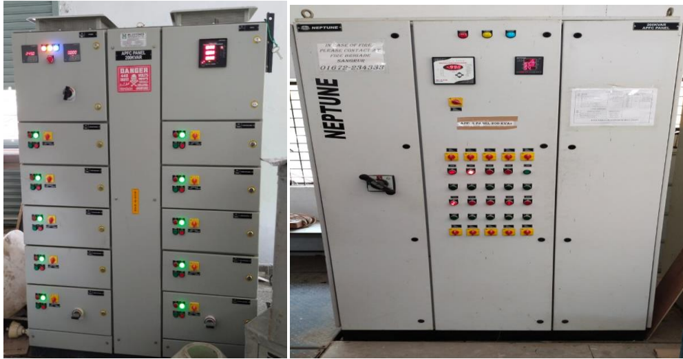
Fig. 3.1: APFCR Panel at ESS-I and ESS-II
