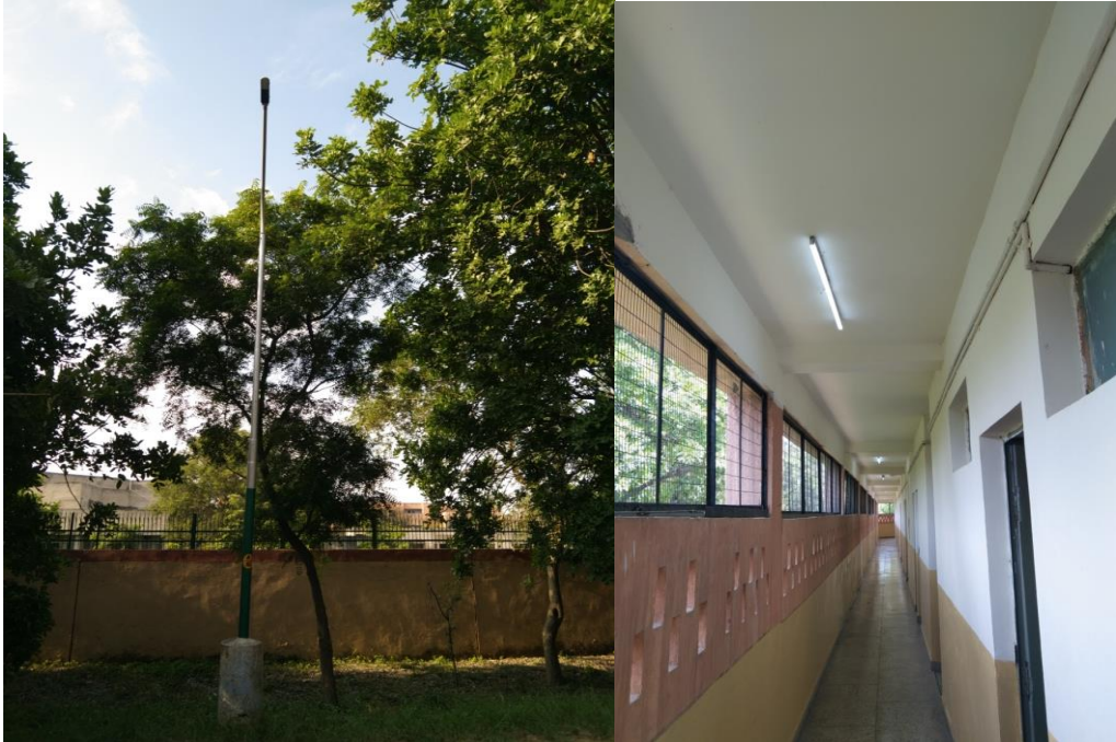
Fig.3.3: LED Fixture (Street Light, Road-A Near H Pole)/ LED Fixture in Girls Hostel No.1, FF (Corridor) Near Room No. 231
