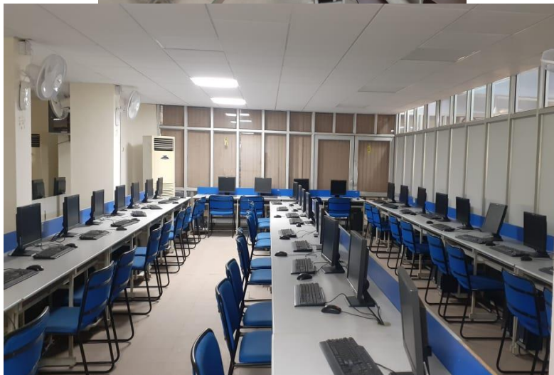
Fig. 3.6: LED Fixtures in Smart Classrooms (Science Hall 4, TF)
